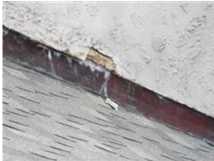
Photo 7-6 Top coat damage could allow water to penetrate behind the flashing.
