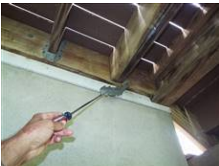
Photo 5-3 This bracket is broken.
