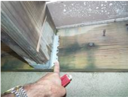
Photo 5-1 Numerous brackets are missing nails. Every nail hole should have the correct sized nail installed. Here and next photo are but two examples.
