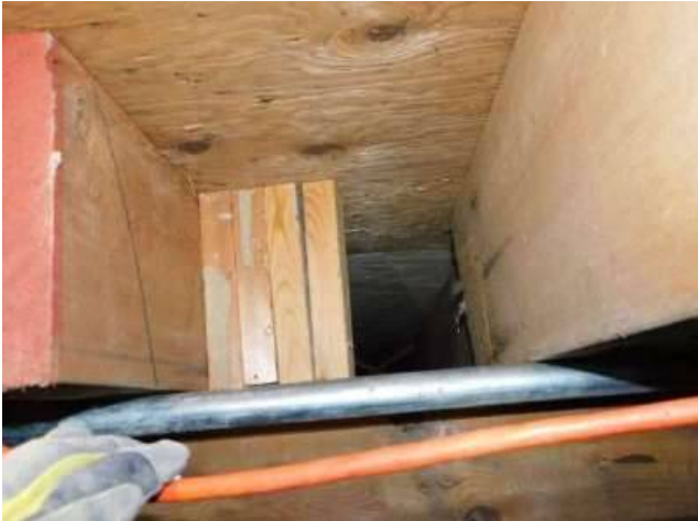
Photo 27-3 Here and the next photo are also the left side but viewed from the street side of the main beam.
