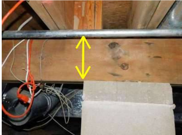
Photo 27-4 One can see that the load is not centered above the column. This is the same as seen in Photo27-2 but from the opposite direction.
