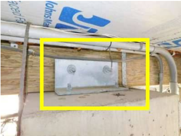
Photo 28-1 This is an example of a post and beam tie seen on another Jersey Shore home.
