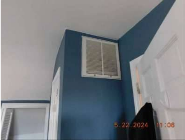
Photo 61-3 Second floor filters for the AC are located behind these return grills. Here and the next 2 photos.
