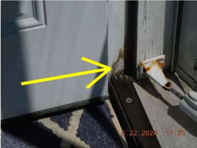
Photo 25-3 The previous photo's damage may be associated with the staining seen here.
