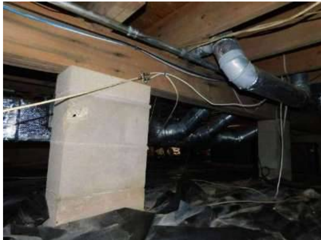
Photo 28-2 No such post and beam ties seen at this location.
