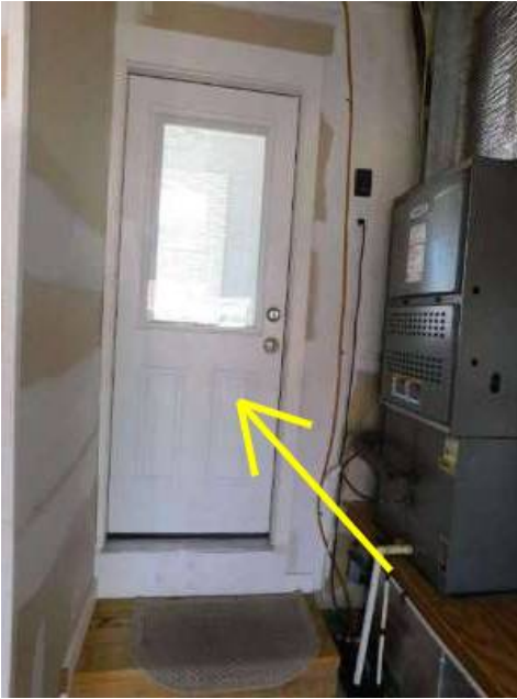
Photo 33-1 The glass may disqualify this as being a fire rated door.
