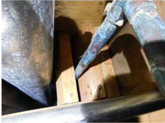
Photo 27-6 However, the inconvenience of the pipe and duct resulted in the structural construction to be changed. This may not be how it was intended. There are three added wood blocks vs. 4 on the other side (First few photos).
