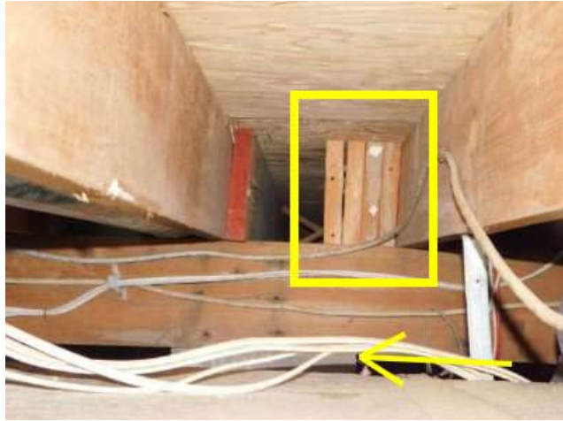
Photo 27-2 The edge of the concrete block column is highlighted with the arrow. One can see that 2 of the 4 blocks above are not over the column.
