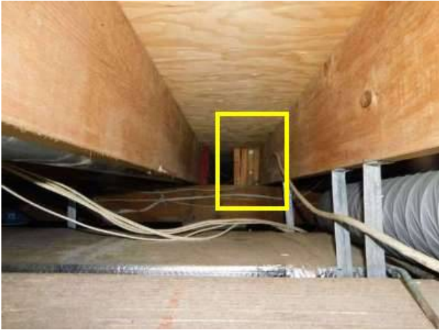
Photo 27-1 Here and the next photo are the left side of the span, when standing inside the house, and viewed from the canal side of the main beam.
