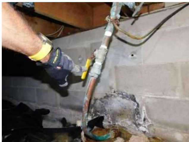
Photo 50-2 Main, water shut off valve.
