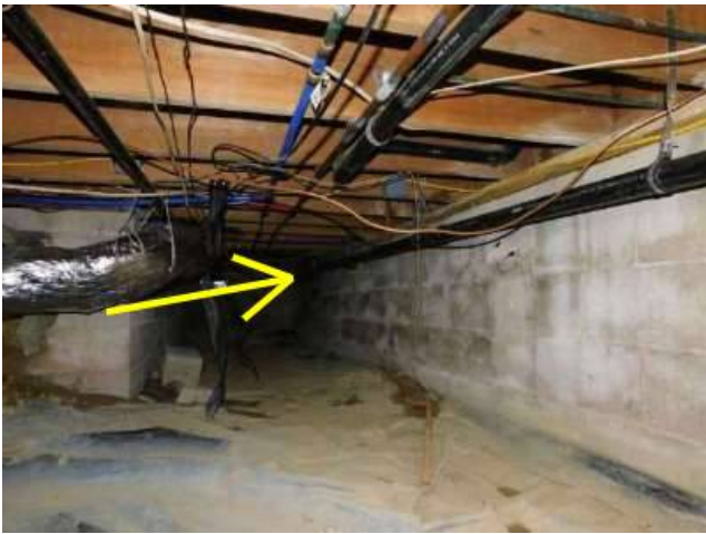
Photo 26-1 If one goes straight back from the crawl space hatch they will enter this area. The following photos were taken back there (Arrow).
