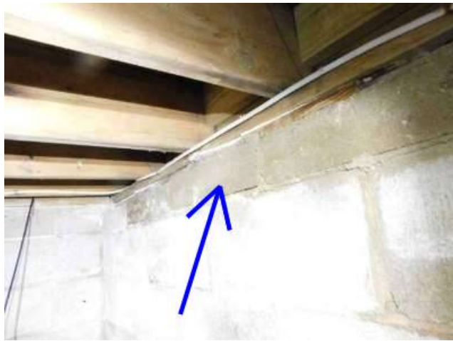
Photo 26-2 The concrete block is wet.
