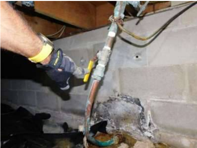
Photo 47-1 Main, water shut off valve.
