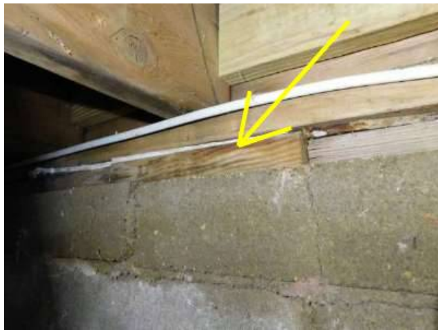
Photo 26-4 The wood sill plate was also measured. It's in contact with the concrete block below so it will absorb the moisture in the block.
