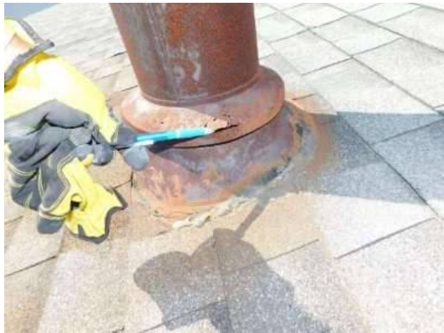
Photo 19-2 There are gaps or holes in the rusted metal.
