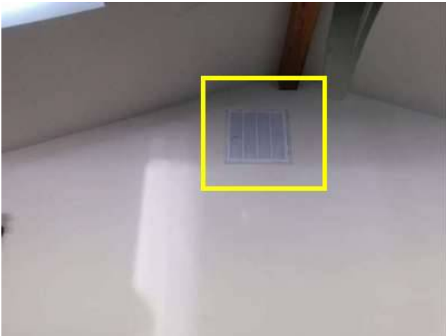
Photo 87-3 This high return for the smaller AC is efficient in that it draws the warmest air in the room back to the AC's evaporator coil for cooling.
