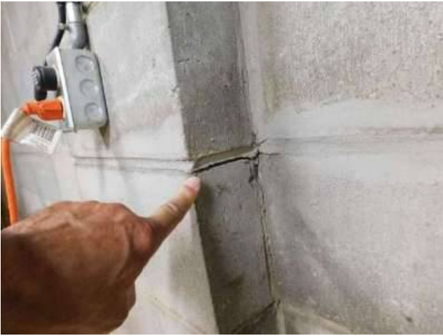
Photo 15-1 A gap at one of the buttresses along the back wall was the first indication of a horizontal crack.
