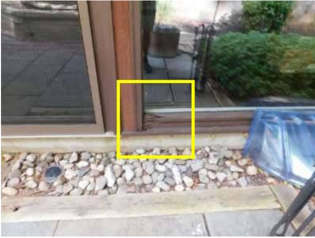
Photo 1-1 Close up of this area in the next photo.
