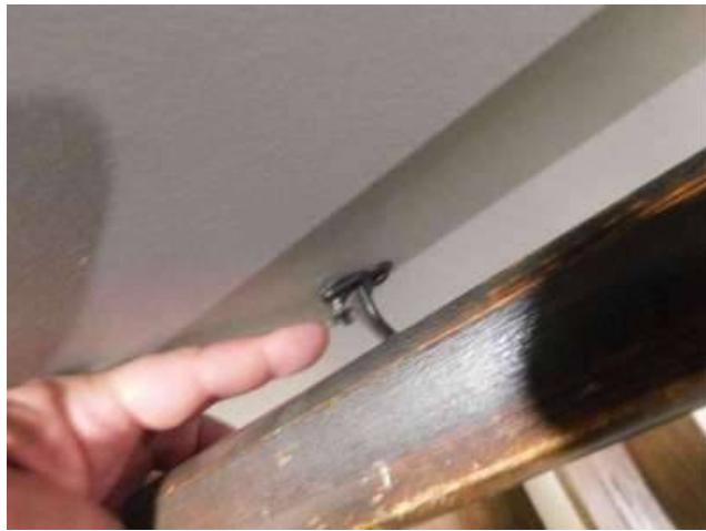
Photo 116-2 One of the screws holding the handrail in place has begun to come out.
