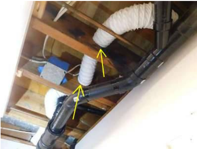
Photo 37-3 The holes made to route the exhaust duct may be too large for the joists. "The maximum hole diameter is 1/3 of the depth of the joist."
