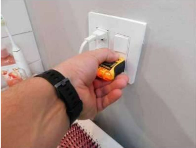
Photo 49-5 This and the following photo were taken in the master bathroom. The right half of the outlet is not GFCI protected but the left half is.
