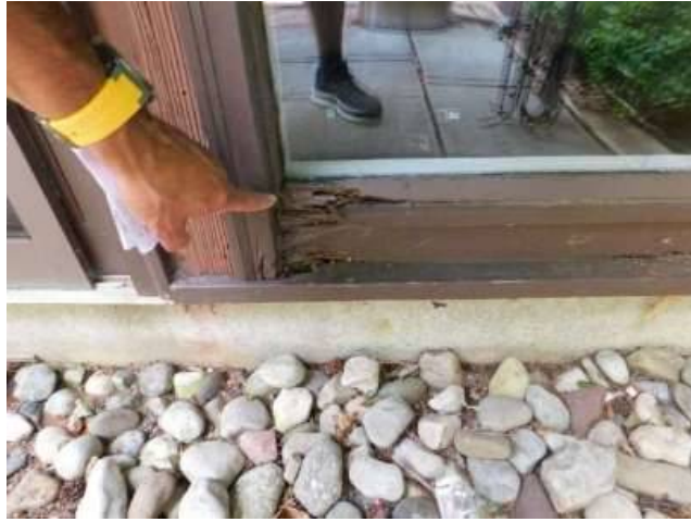
Photo 1-2 Carpenter ant damage identified by the WDI inspector.
