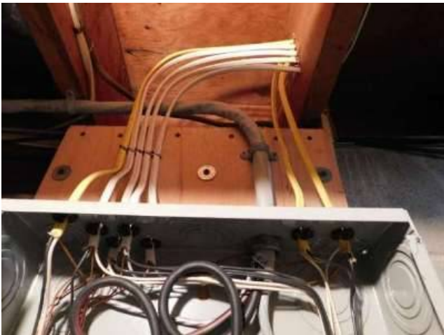
Photo 51-1 Notice the difference between how the 5 cables on the left (Next photo) are secured vs. the 2 cable on the right (Last photo).
