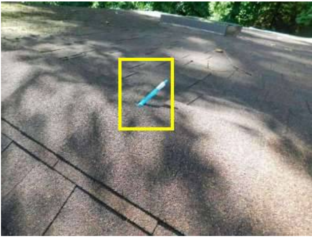
Photo 25-1 Seen in the ridge on the bedroom side of the roof. Close up of this area in the next photo.
