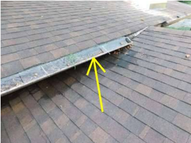
Photo 26-1 Debris and weeds seen in the gutter.
