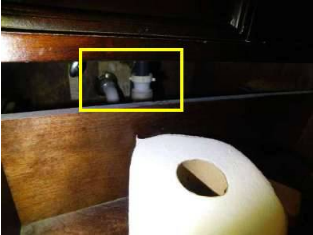
Photo 101-1 Close up of this area in the next photo.
