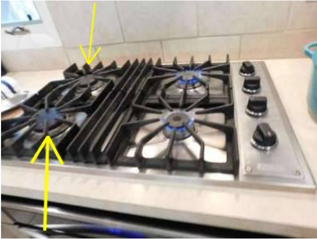
Photo 100-1 There was no response from these two burners.
