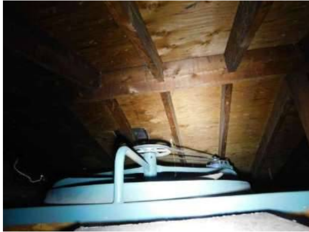
Photo 35-2 This is the whole house fan assembly in the attic.
