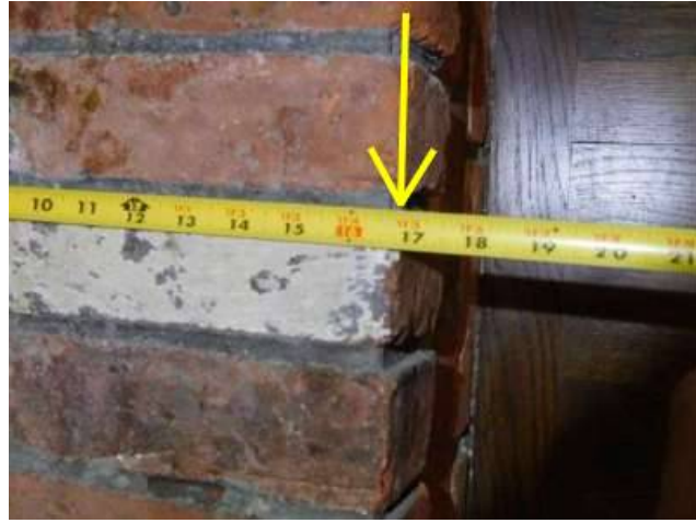
Photo 93-4 This photo is looking down on the hearth. The floor can be seen on the right side of the photo. The hearth is less than 20 inches from the fireplace.
