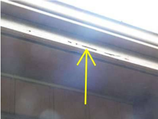
Photo 1-3 Carpenter bee damage seen at the front eave.
