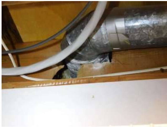
Photo 37-2 The joist appears to have been severed.
