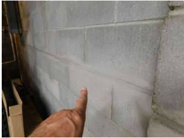
Photo 15-2 The same, horizontal mortar line has clearly been patched. A hairline horizontal crack can also be seen a couple of courses of blocks above.
