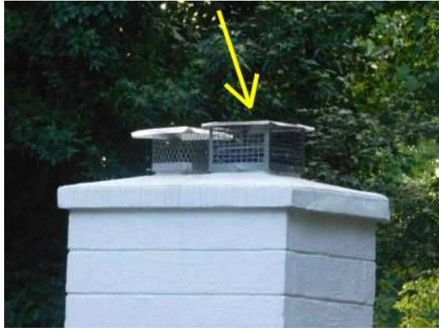
Photo 95-2 The masonry chimney at this location has a rain cap which is appropriate for a wood burning fireplace but not for venting gas appliances as we have here.
