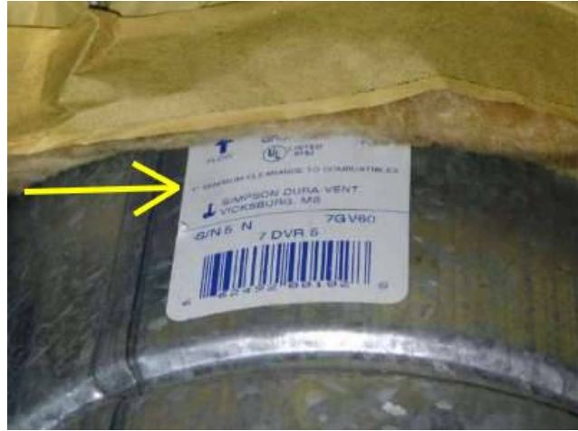
Photo 55-2 Label seen on the vent. "1" minimum clearance to combustibles." The insulation is not combustible but the paper around it is.
