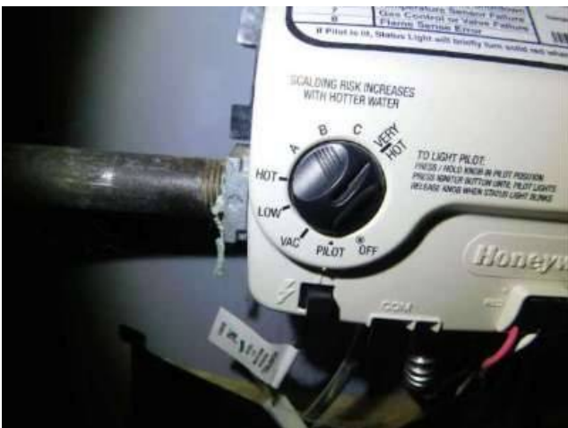
Photo 56-7 Upon arrival, the water heater was set to the manufacturer's "VERY HOT" setting. As noted on the thermostat, "SCALDING RISK INCREASES WITH HOTTER WATER".
