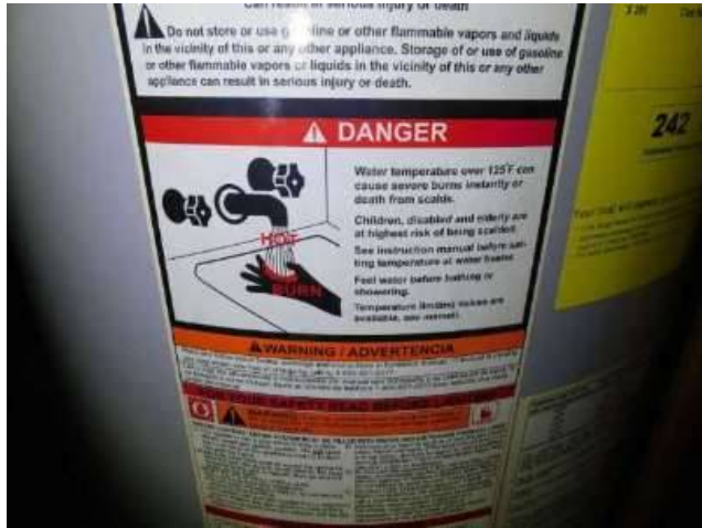
Photo 56-6 Warning label seen on water heater.
