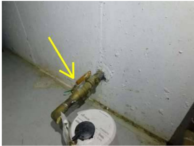
Photo 53-2 Water shut off valve.
