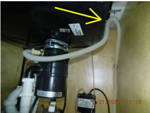
Photo 74-1 This is an example of a high loop from a DIFFERENT property. No high loop was seen for THIS property.
