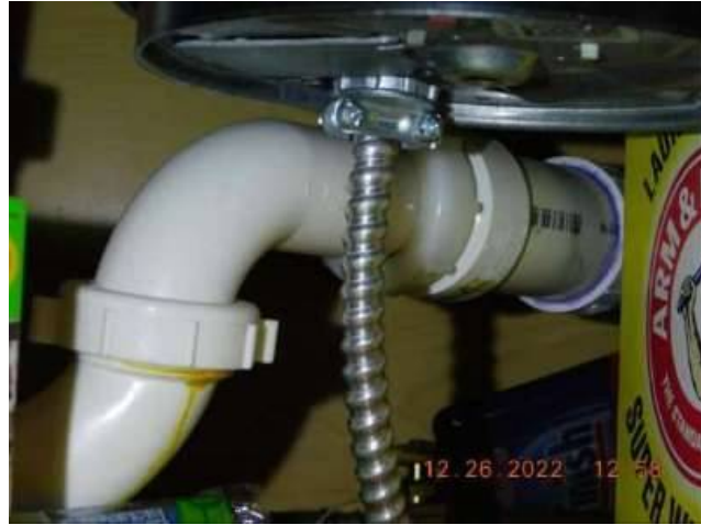
Photo 73-4 This is an example of armor clad wiring from a DIFFERENT property.
