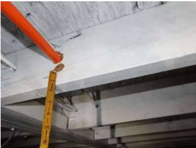
Photo 34-3 Holes must be 2 inches or more from the joist's edge as noted in one of the bullet points above. Here and the next 2 photos are examples of holes that are less than 2 inches from the bottom edge of the joist.
