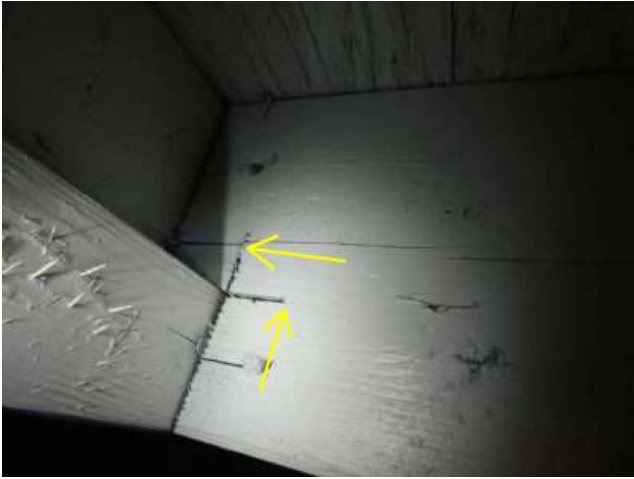
Photo 34-1 Numerous joists have been cut to create the needed notches to hang from the ledger board. The cuts made are significantly longer than need be. This weakens the joists. Another item in this section shows a number of split joists. The split almost always starts at these poor cuts.
