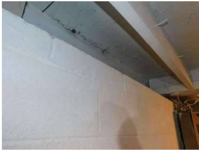
Photo 33-4 Here and the next photos are along the wall with the electrical panel.
