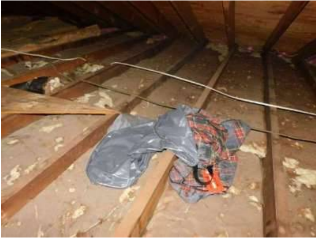
Photo 24-1 Here and the next 3 photos are probably original insulation. Quite compressed, thin and ineffective as an insulating barrier.
