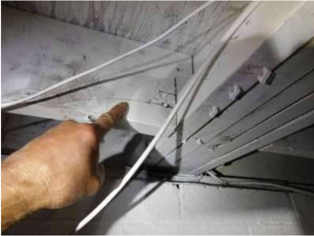
Photo 37-1 Some of these splits appear to be associated with the large cuts that were made to create the notches as noted above in this section.
