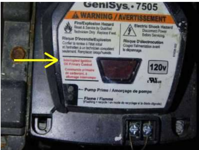
Photo 74-3 "Interrupted ignition oil primary control"
