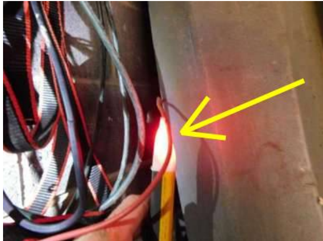
Photo 45-2 Exposed, insulated conductors. The voltage detector confirms that the exposed wires are energized.
