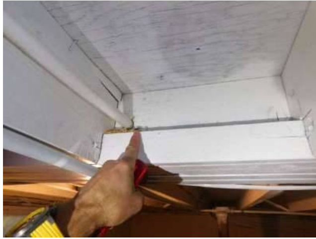
Photo 34-6 In this case, a beam is drilled. While joists can be drilled within reason, beams should never be modified, drilled or notched.
