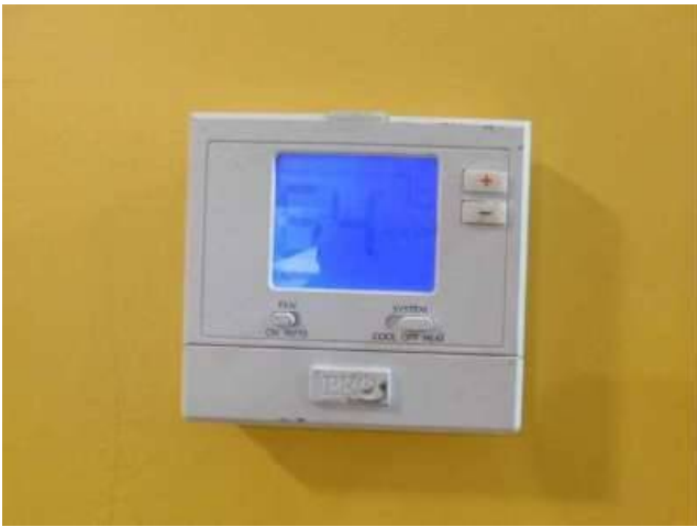
Photo 74-1 Upon arrival the thermostat was calling for heat but the boiler was not running.
