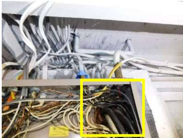
Photo 42-4 Rusted components inside Panel A. Findings will likely show that water is using the main electrical cable as a conduit to enter, and damage, Panel A.
