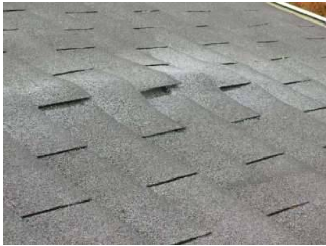
Photo 16-2 There is a distinct deformity in the roof surface. Requires repair by a qualified roofing contractor.
