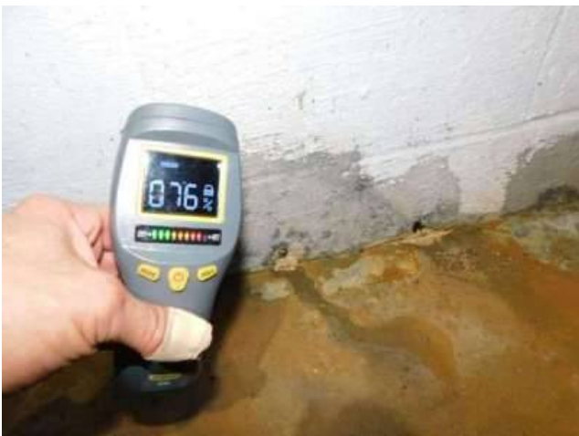
Photo 36-3 While it's obvious that there's moisture, the moisture meter confirms that.
