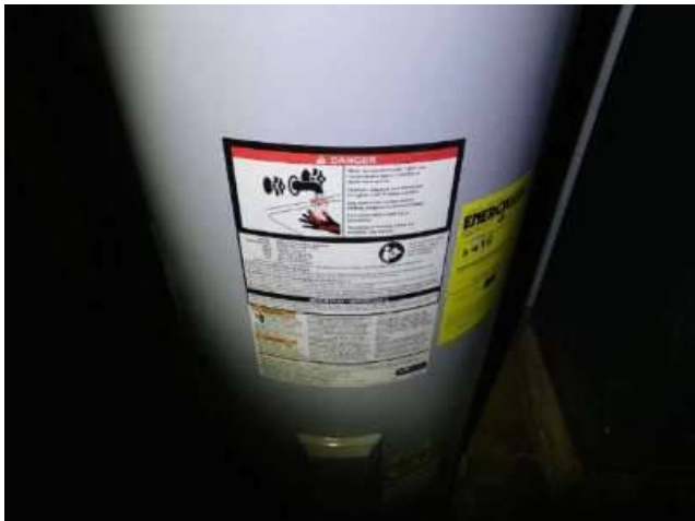
Photo 70-1 Warning label seen on the water heater regarding hot temperatures.
