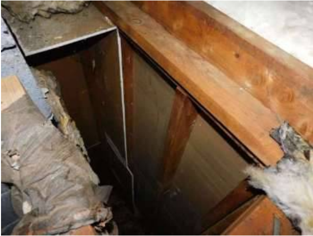
Photo 24-5 Interior, living space walls are not insulated and exposed to the extreme temperatures in the winter and summer. This increases energy costs as cold temperatures easily radiate into the living space in the winter and very hot temperatures radiate into the living space in the summer.
