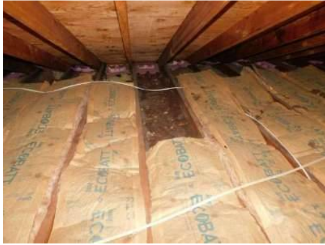
Photo 24-10 Some insulation has been added but sections are missing.
