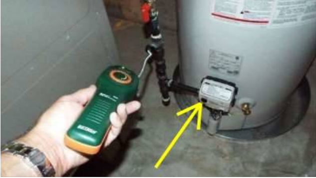
Photo 26-1 This dial should be adjusted. It's currently set, by the occupant, to higher than the labeled, "HOT" setting. Recommend adjusting it downward to the HOT setting at your day-of-closing walk through.
