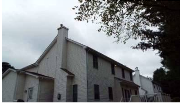
Photo 12-6 The upper, back side was inaccessible for visual inspection.
