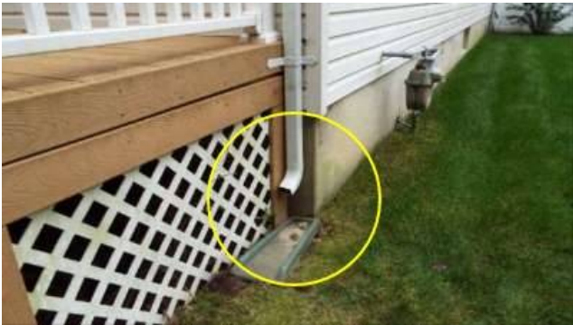
Photo 10-1 Water is deposited too close to the foundation wall.
