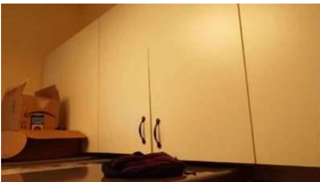
Photo 38-1 The right side of this set of cabinets in the Laundry room appears to be falling off the wall and should be properly secured.
