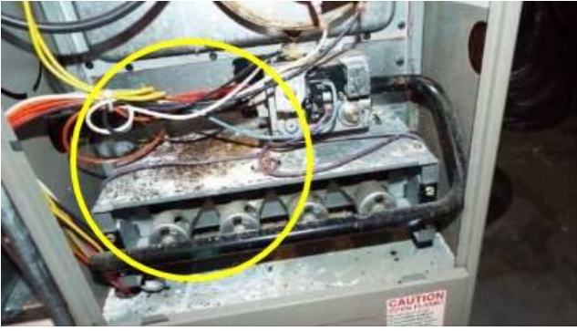
Photo 30-1 There's an abundance of rust particles and debris in the furnace which suggests that it hasn't been professionally serviced for years.
