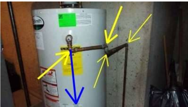
Photo 27-1 The Monroe Twp, "Final" inspection sticker is on the water heater. Typically the drain goes straight to the floor as indicated by the blue arrow.
