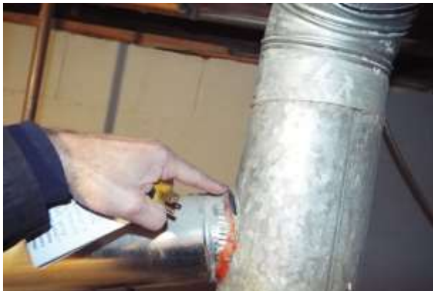
Figure 1 - There's a large gap where exhaust will leak into the living space.
