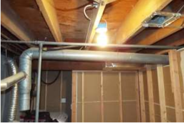
Figure 2- The horizontal flue seen in this photo is pitched down. It's lower on the right than it is on the left.
